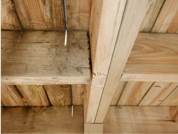
Corroded nails and separation
